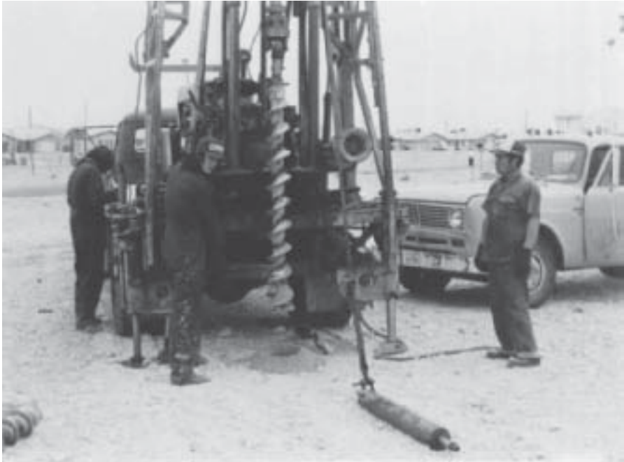
Figure 10.3 Drilling with continuous-flight augers (Courtesy of Danny R. Anderson, Danny R. Anderson Consultants, El Paso, Texas)
