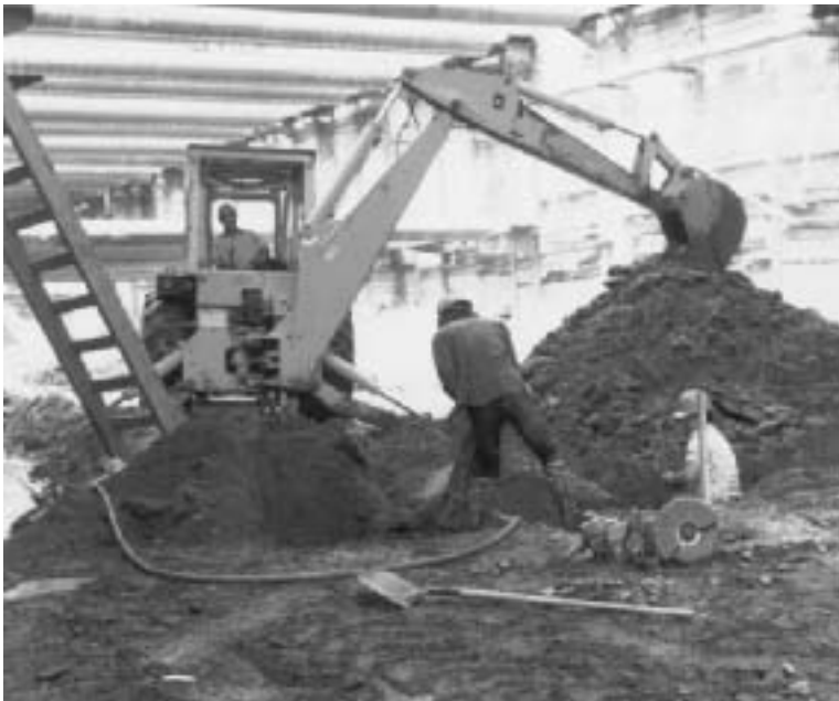
Figure 13.20 Braced cut in the construction of Washington, D.C. Metro (Courtesy of Ralph B. Peck)
