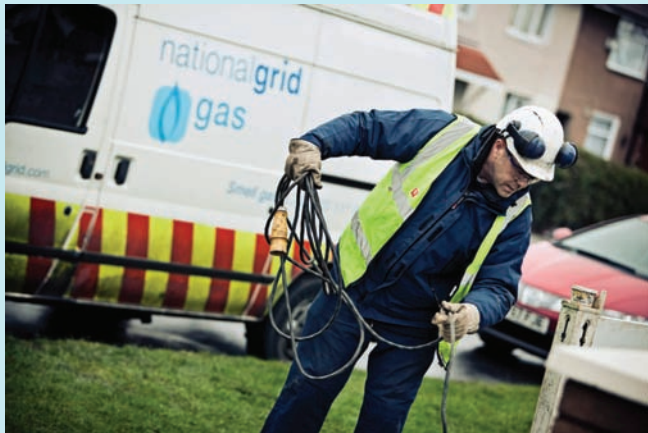
Source: National Grid
